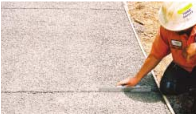
Gainesville, Georgia employee places expansion joint in pervious concrete sidewalk near government offices in May 2003.
