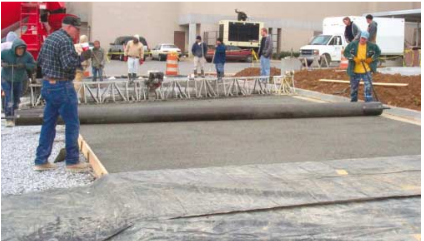
Pervious concrete is placed in a parking lot at a hospital in Morristown, Tennessee. January placement required blankets instead of plastic sheets to retain moisture and heat of hydration.
