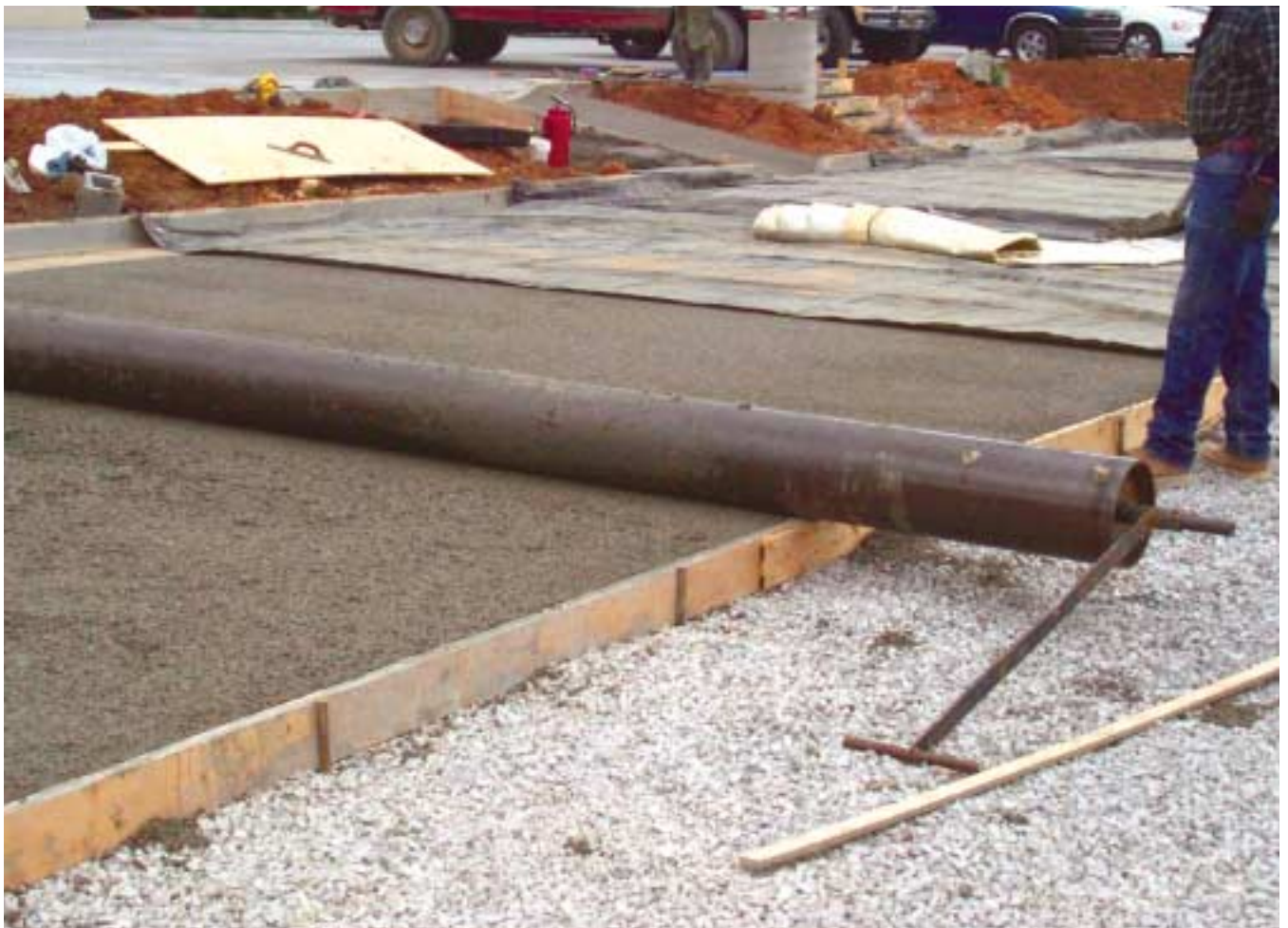
Pervious concrete is lightly compacted after placement using a static roller. The site is a Morristown, Tennessee hospital parking lot.
